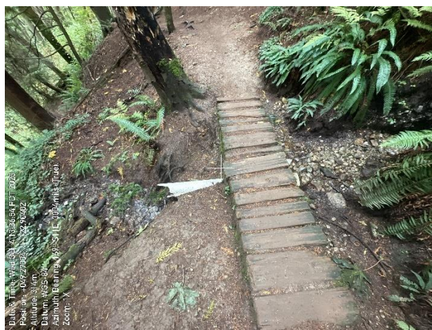
Degraded culvert under boardwalk. Signs of vegetation damage surrounding tributary and trail.
