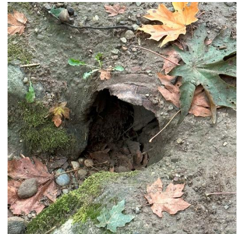
Severely degraded culvert in need of repair.
