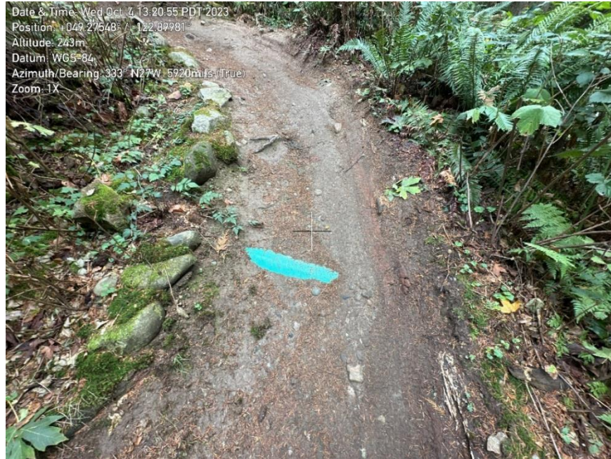
Photo 7: Erosion and poor trail maintenance. Surface water infrastructure can be seen within the middle of the trail, but fully embedded under the soil on the inlet and outlet.
